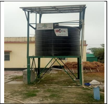
Fig: Solar Based pump for drinking water
