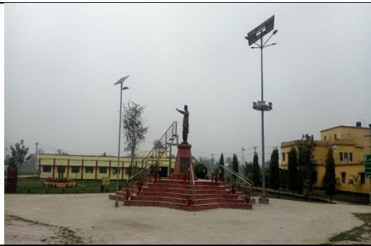
Fig: Solar based street light system
